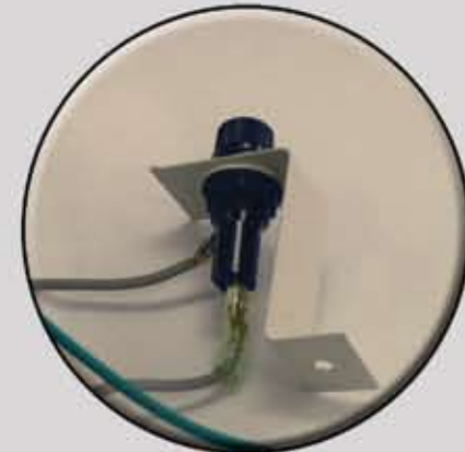
2. Low Voltage Fuse Protection
